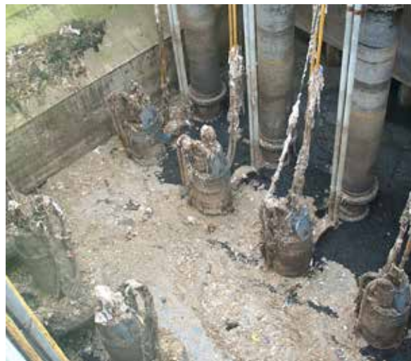
Pump station with accumulation of floating debris.
