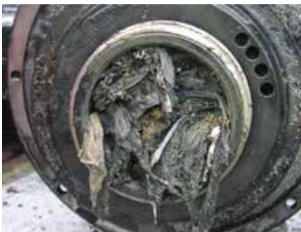
A clogged pump.
