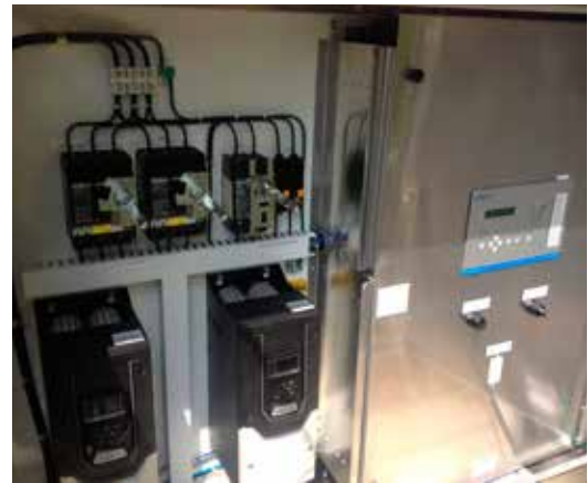
The pumps are monitored and controlled by a Flygt AquaView SCADA system.
