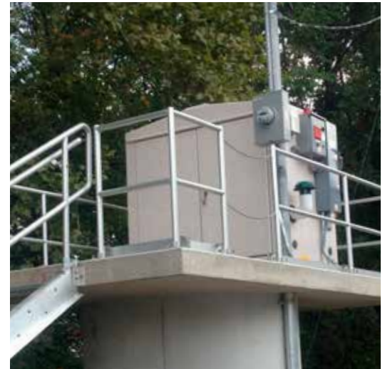
The Gilman Avenue Lift Station
