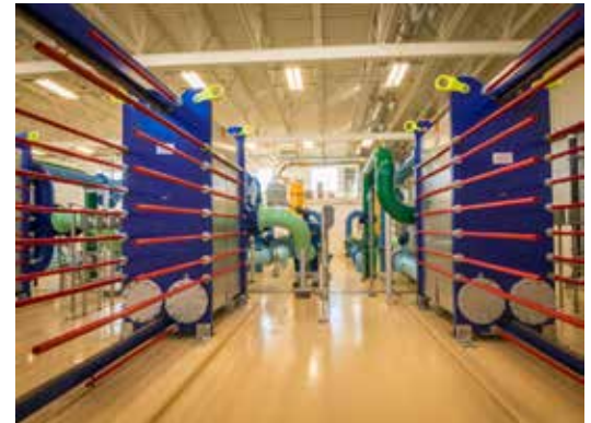
Plate and frame heat exchangers heat and cool the water within the NIC piping loop.
