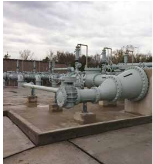
New lift station in Houston, TX includes six Flygt CP3356, 280-horsepower submersible pumps
