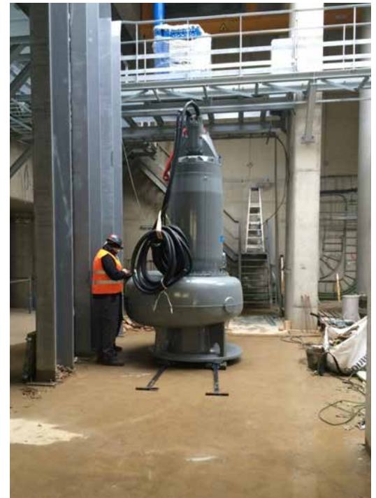
Flygt CP 3800 - 55 MGD pump ready to be installed
