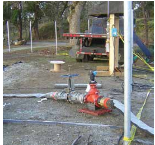
The combination valve (vacuum breaker & air release) and a 6" gate valve to manage the flow.
