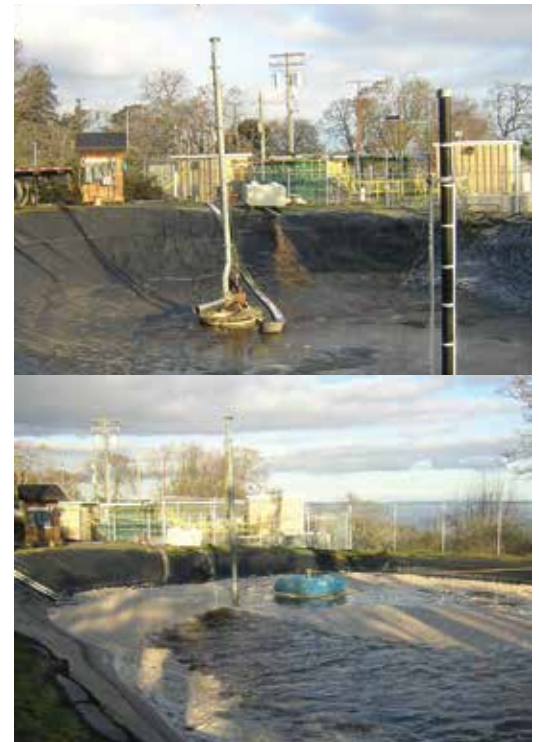
The temporary lagoon where the Flygt Jet Aerator, the N 3153 submersible pump and the flotation module were installed.
