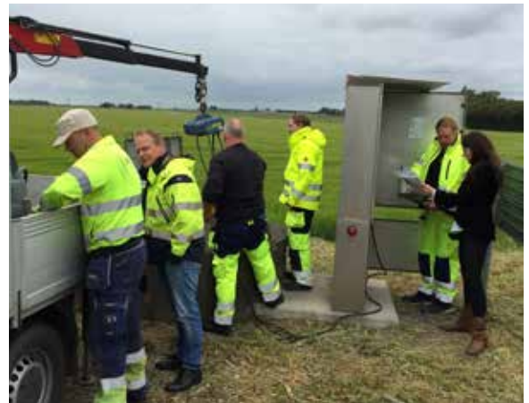
Installation of Flygt Concertor at Lomma Municipality.
