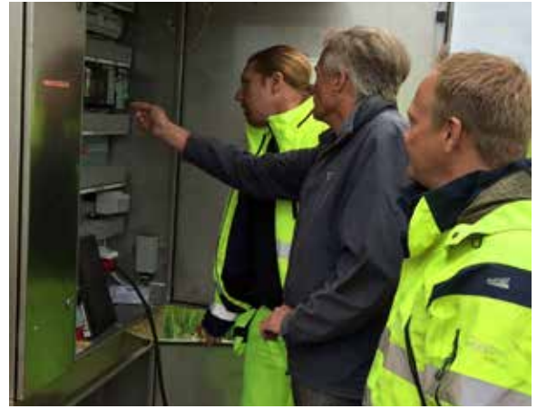
Anders Sjöström (first from the right), Manager at Borgeby treatment plant, testing the Flygt Concertor system with the support of Xylem staff.
