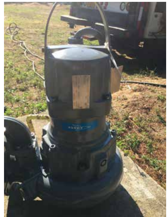
Concertor trial pump ready to be installed
