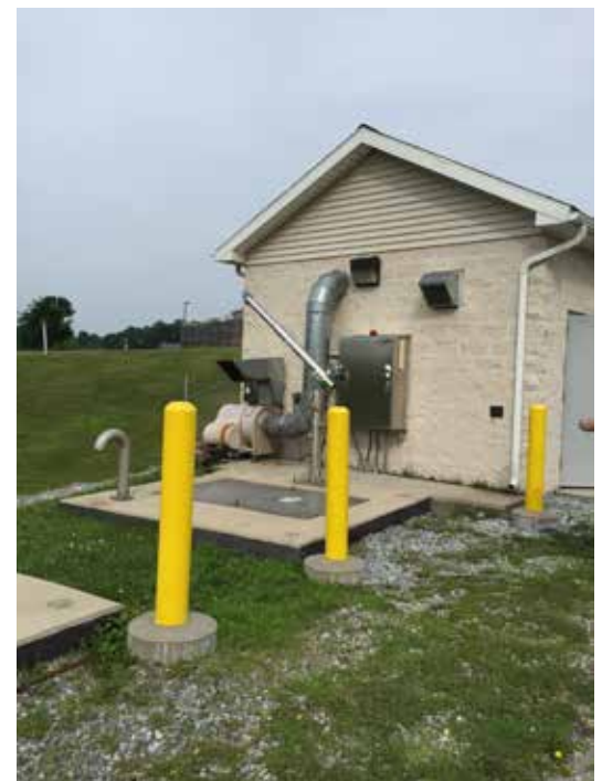
Chester County Prison pump station
