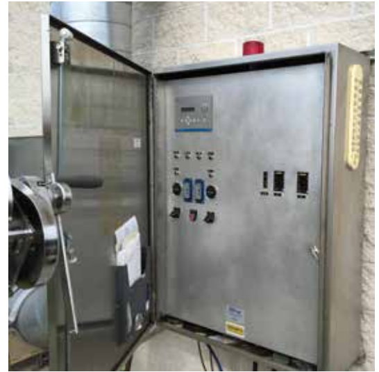
Existing control panel can be reduced in size with Concertor solution.
