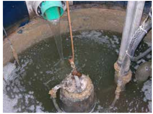
Hospital discharge from blue pipe is transferred to WWTP by two pumps.
