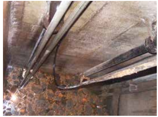
Inside the lift station.
