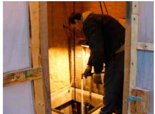
Final rinse for the N-pump.
