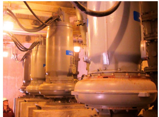
The new N-pumps installed.
